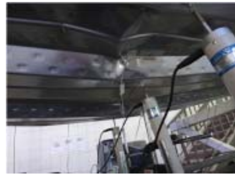
Fig. 5. Local buckling at the top flange of the profiled steel sheeting (experiment)
